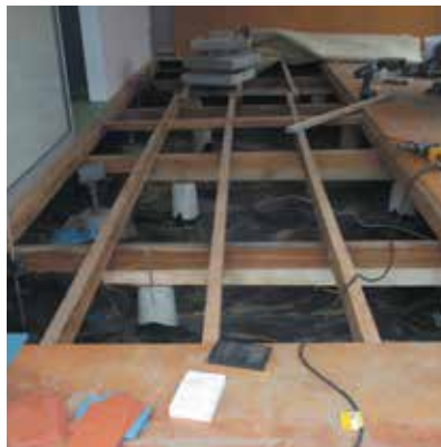
02: Where lift was over 100mm, piles were packed with an extra bearer spanning at least two piles
