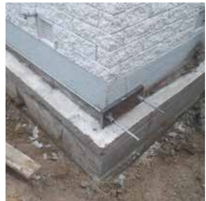
03: Tension bars pulled foundation together closing up cracks
